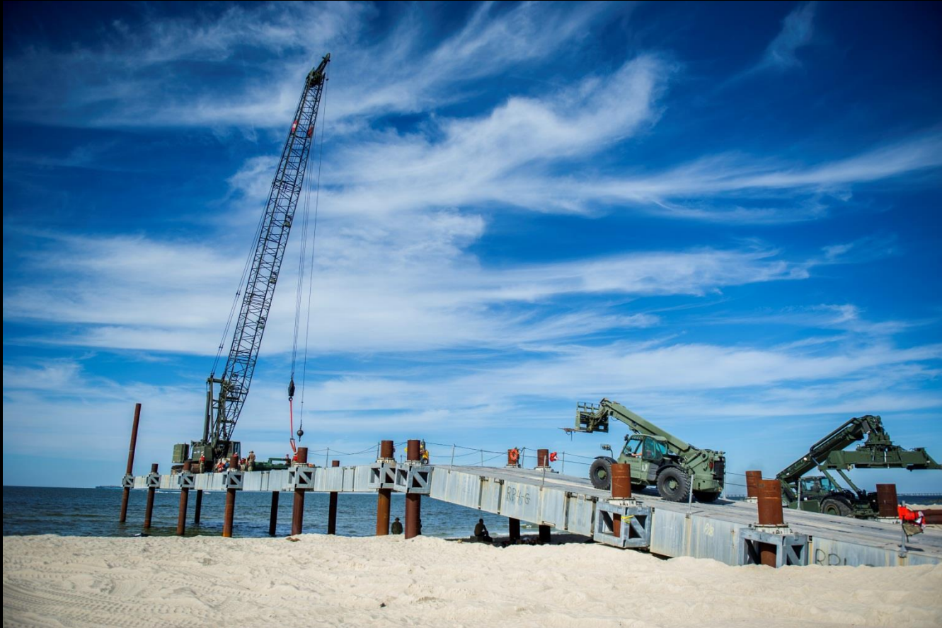
End of day 9 (15 Aug) at PHIBCB TWO's ELCAS build, Anzio beach JEB-LCFS. (U.S. Navy Photos by Engineering Aide 2 nd Class Larry Winer.)
